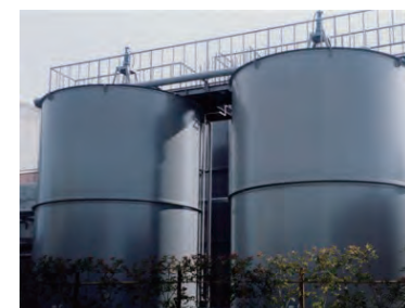
Continuously Self-Cleaning Fixed Film Bioreactor
