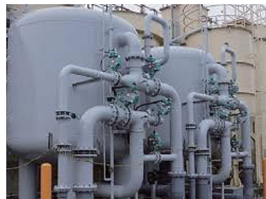
Sand Filtration System
