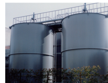
Continuously Self-Cleaning Fixed Film Bioreactor
