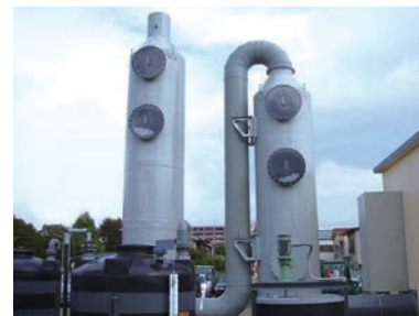
Odor Control Wet Scrubbing Tower
