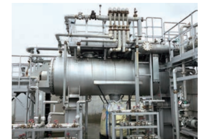
Vacuum-Type Sludge Dryer
